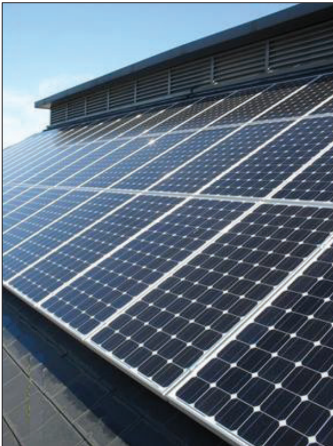
Solar panels mounted on a roof
